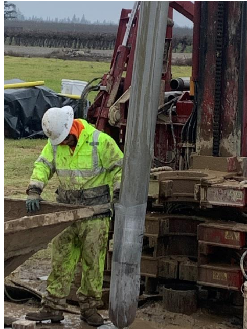
Photograph 7. Drilling on Monitoring Well Soil Boring (collection of continuous cores from sonic core barrel)
