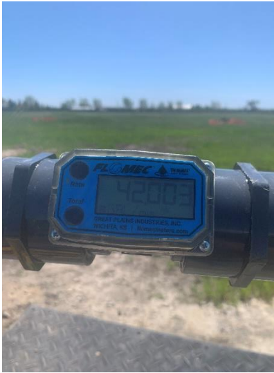
Photograph 11. Flow Meter and Totalizer (both in same instrument)
